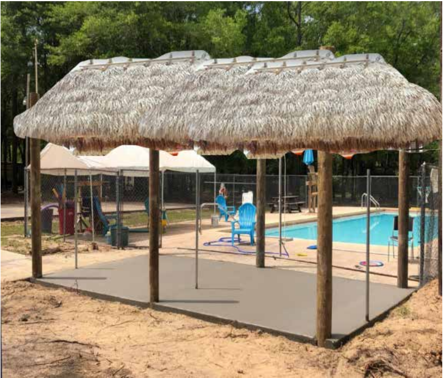
Tiki Hut that will provide shade at one end of the Pool.
